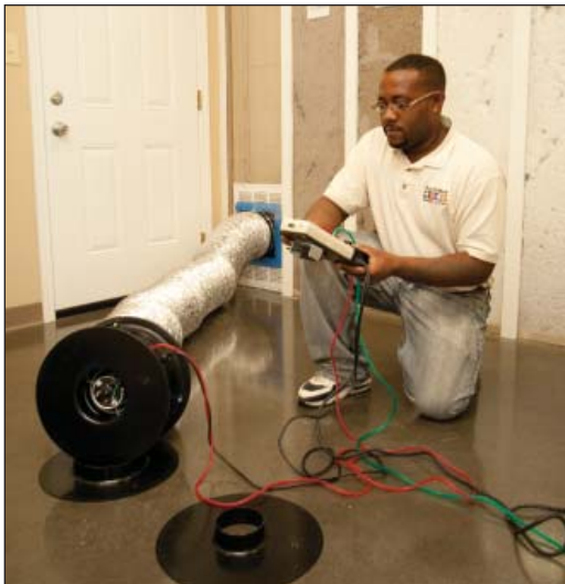
This technician is performing a duct leakage test that ensures the integrity of the duct system.
